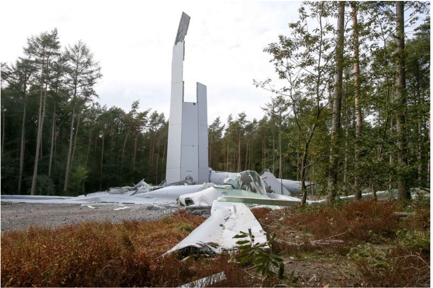
This 784-foot-tall wind turbine in Haltern, Germany, collapsed in 2021. Photographer: TF-Images/Getty Images
